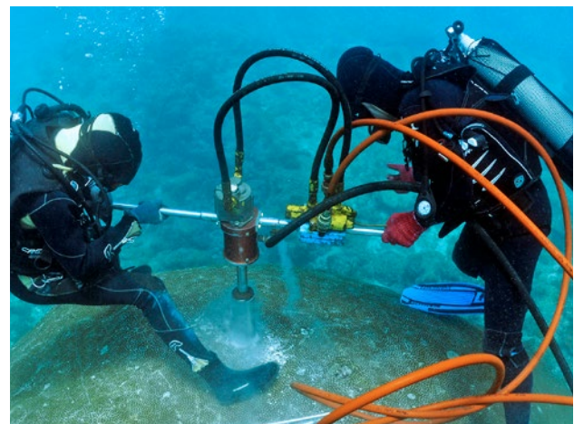
Extracting a coral core: afterwards the hole is filled with underwater cement to protect the coral
